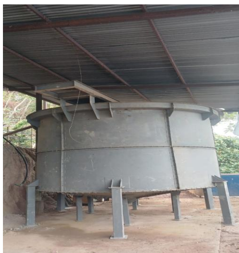
PHOTO 1: NEW THICKENER – SANTA BARBARA PROCESSING PLANT
