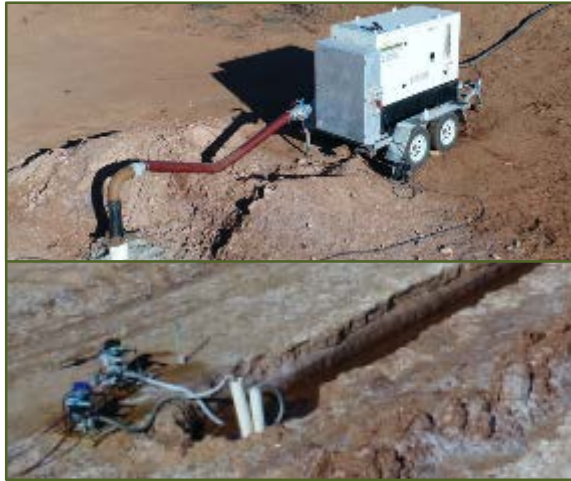
Brine Pumping from Bores and Trenches >120 Million litres successfully pumped to date
